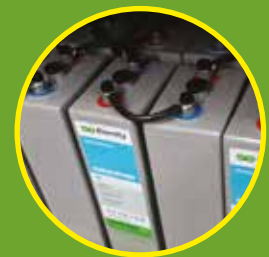
Deep-cycle long life, mainteance free batteries
